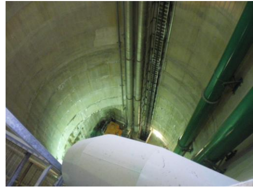
Mt Crosby, 34 metre deep pump well.
